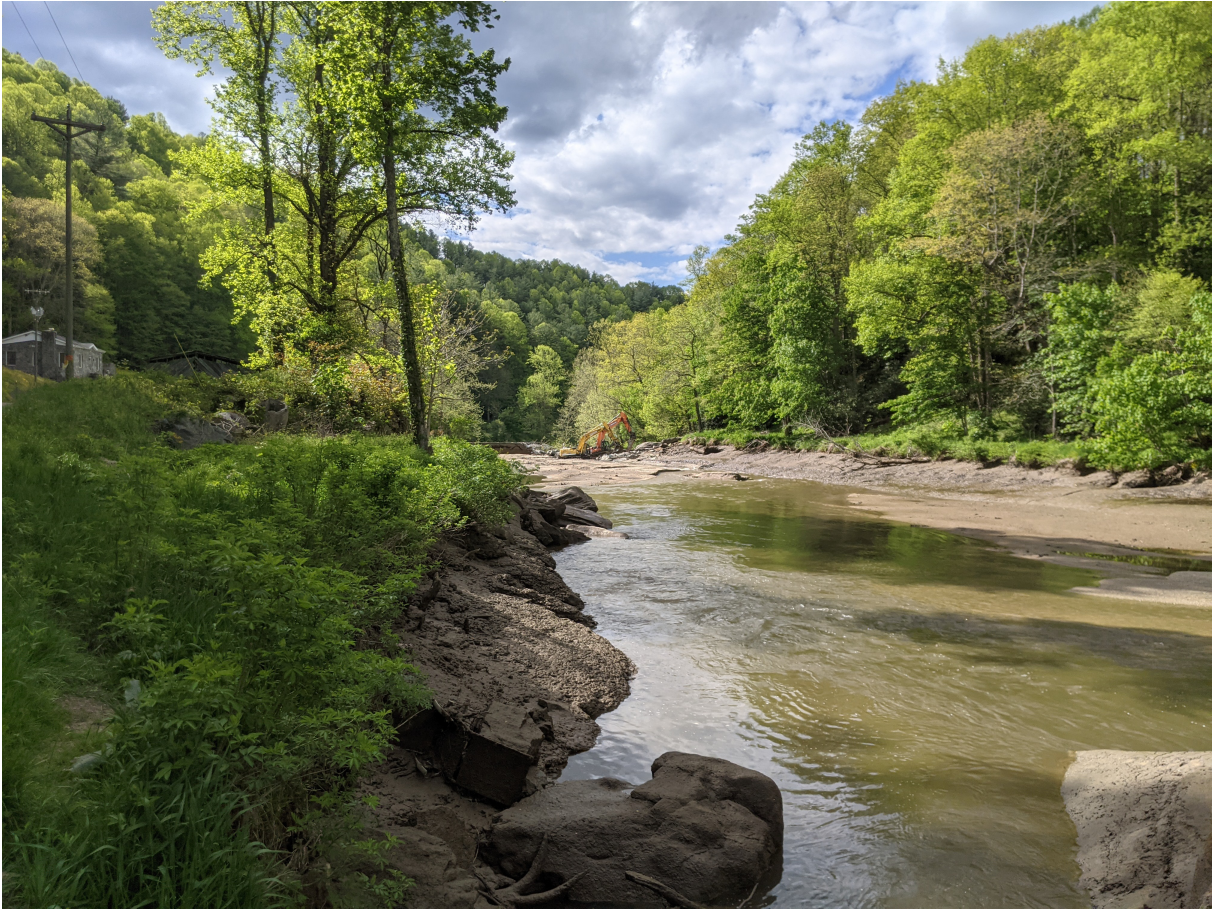
Figure 7: Image of the dam removal as seen from upstream showing the mud and sand bed as it is exposed by receding water within the former impoundment. Image credit to Josh Platt, 2021.
